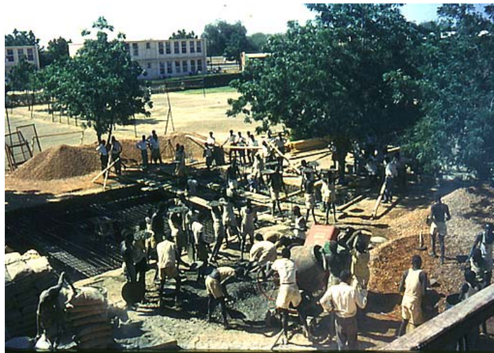
The construction work started for the foundation of Block 12B at Khartoum Technical Institute
